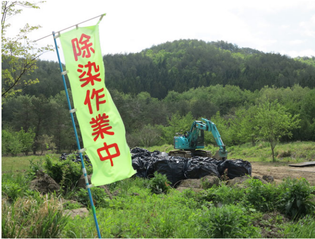
Figure 2. Piles of black plastic bags filled with radioactive soil and debris in Iitate, Japan, 2016. These were by-products of state-sponsored decontamination work. No one knew how to properly dispose of them. [This figure appears in color in the online issue]
